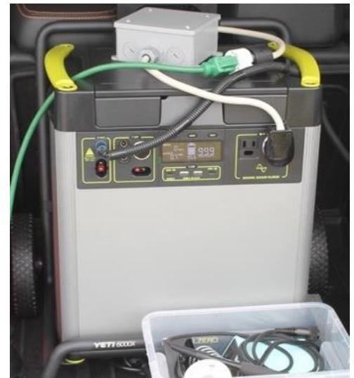
Goal Zero lithium battery units and solar panels for Station 1 (AG7NR)
